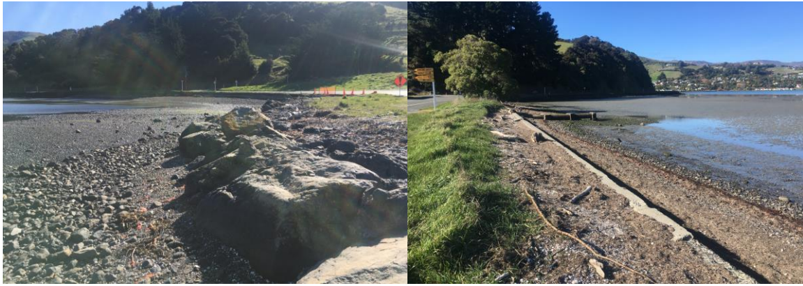
Figure 4.37: Example of protection structures with evidence of scour and overtopping (Duvauchelle Bay).
