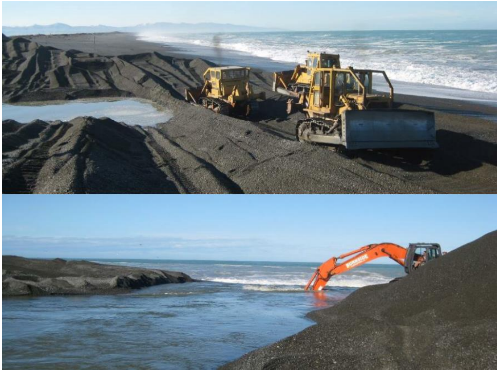
Figure 2.16: Bulldozers removing the 'scab' to make the connection between the cut and sea (top). Excavator working to enlarge the freshly open cut (sourced from Measures et al., 2014)
