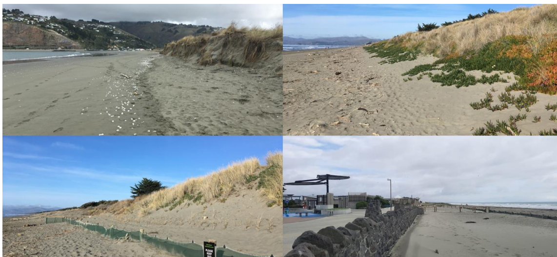
Figure 4.1: Site photos along Christchurch open coast. (Top left) Erosion scarp on Southshore Spit, (top right) vegetated, accreting dunes near Waimairi, (bottom left) dune planting and fencing near Waimairi, (bottom right) seawall at New Brighton.
